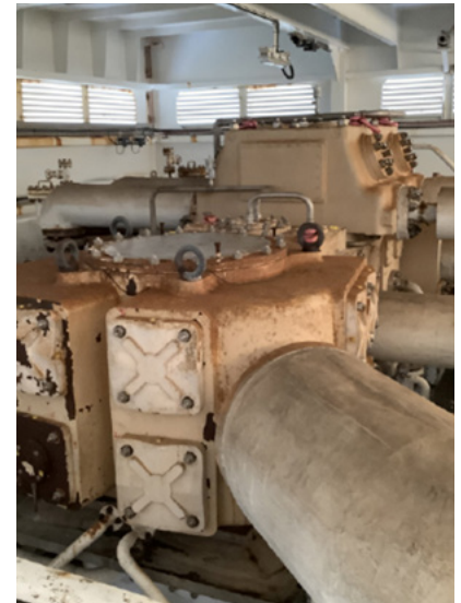
Inspection findings: no maintenance hatch in compressor room.
