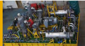
Offshore gas platform Customer: CNOOC Power: 280 kW
