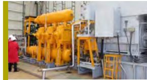
Natural gas pipeline Customer: Sinopec Power: 3 MW
